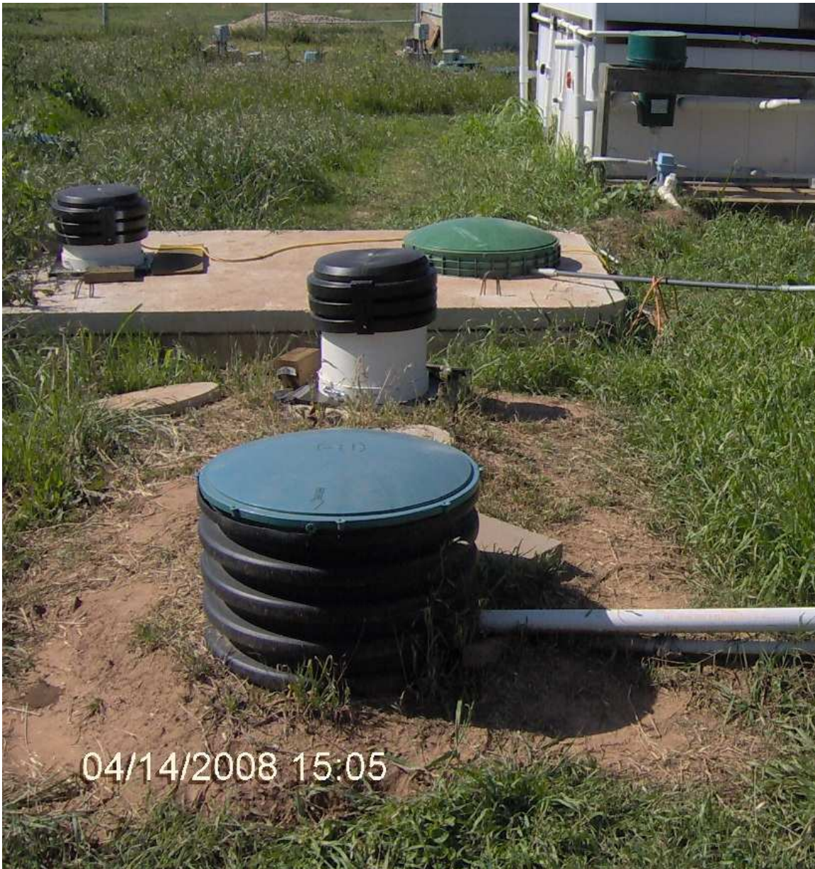
Figure 1. Dosing design. The wastewater flows from the dosing bucket in the upper right to the tank oriented perpendicular to the view and then to the tank oriented parallel to the view in the forefront of the photo. The aerators are located under the black risers and due to the small \frac{1}{4} mm bubble size and low velocity delivery system the air does not appear to mix or agitate the settled solids.
